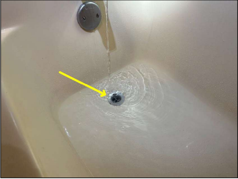
Back hall, bathroom slow drain
