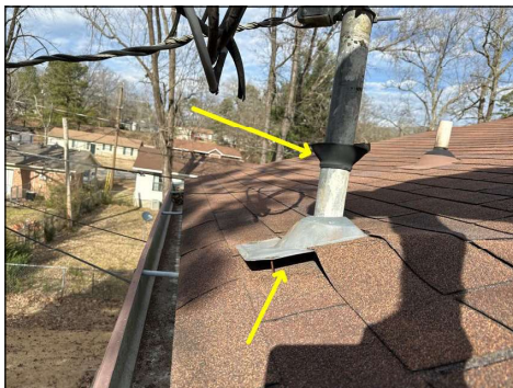
Raised flashing and rubber vent boot
