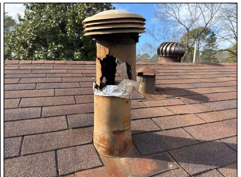
repair/replace damaged/cracked exhaust pipes
