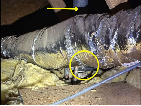
The exhaust pipe was disconnected in attic
