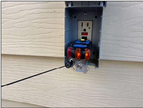
Both exterior back deck receptacles
