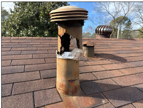
repair/replace damaged/cracked exhaust pipes
