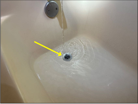
Back hall, bathroom slow drain
