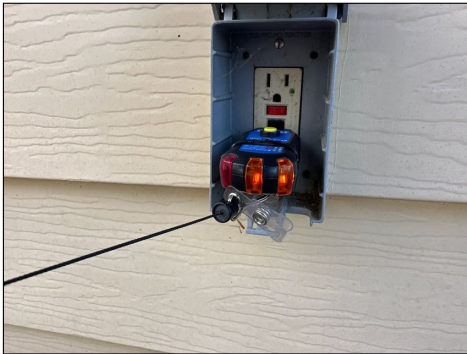
Both exterior back deck receptacles
