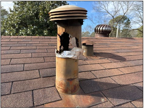
repair/replace damaged/cracked exhaust pipes
