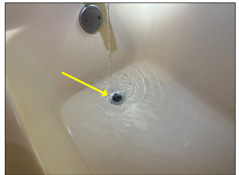
Back hall, bathroom slow drain
